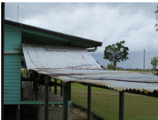
Live Power in Contact with Metal Roofing iron
